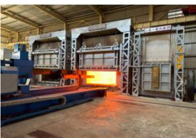
30Ton Natural Gas Heater
